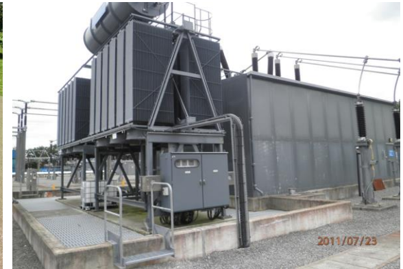
400 kV Power Transformer
